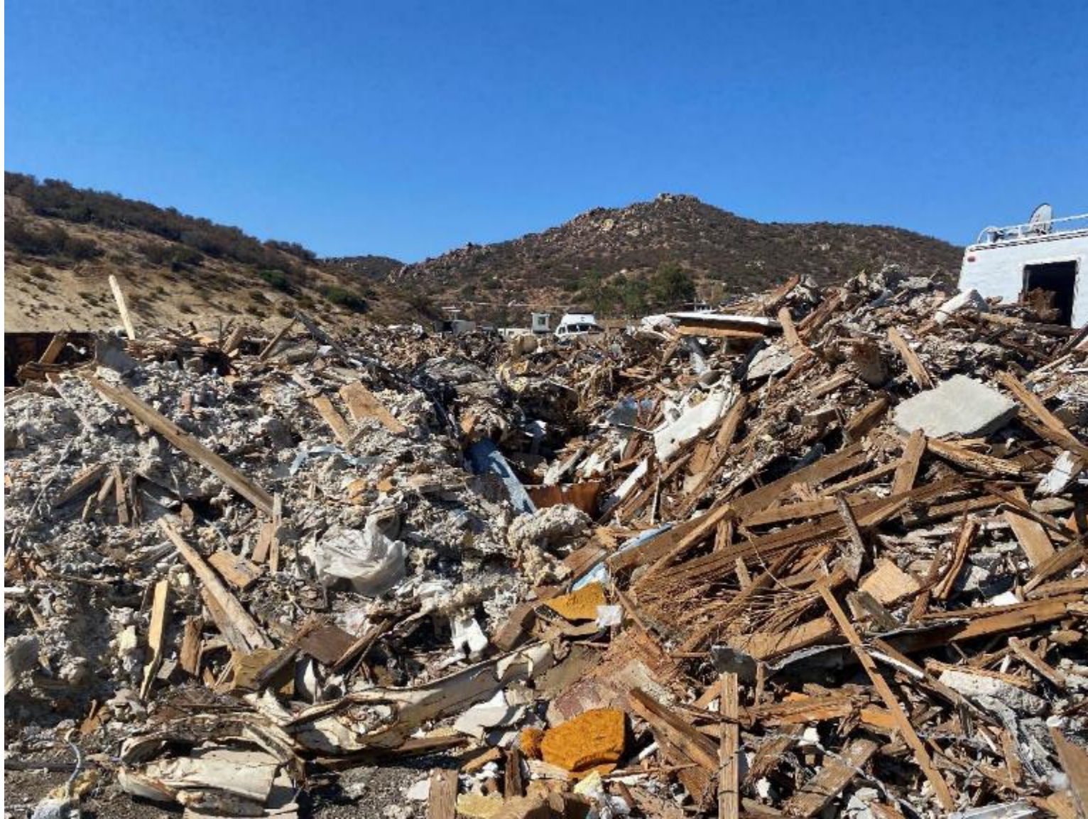
Construction debris, potential asbestos containing materials (ACM)
