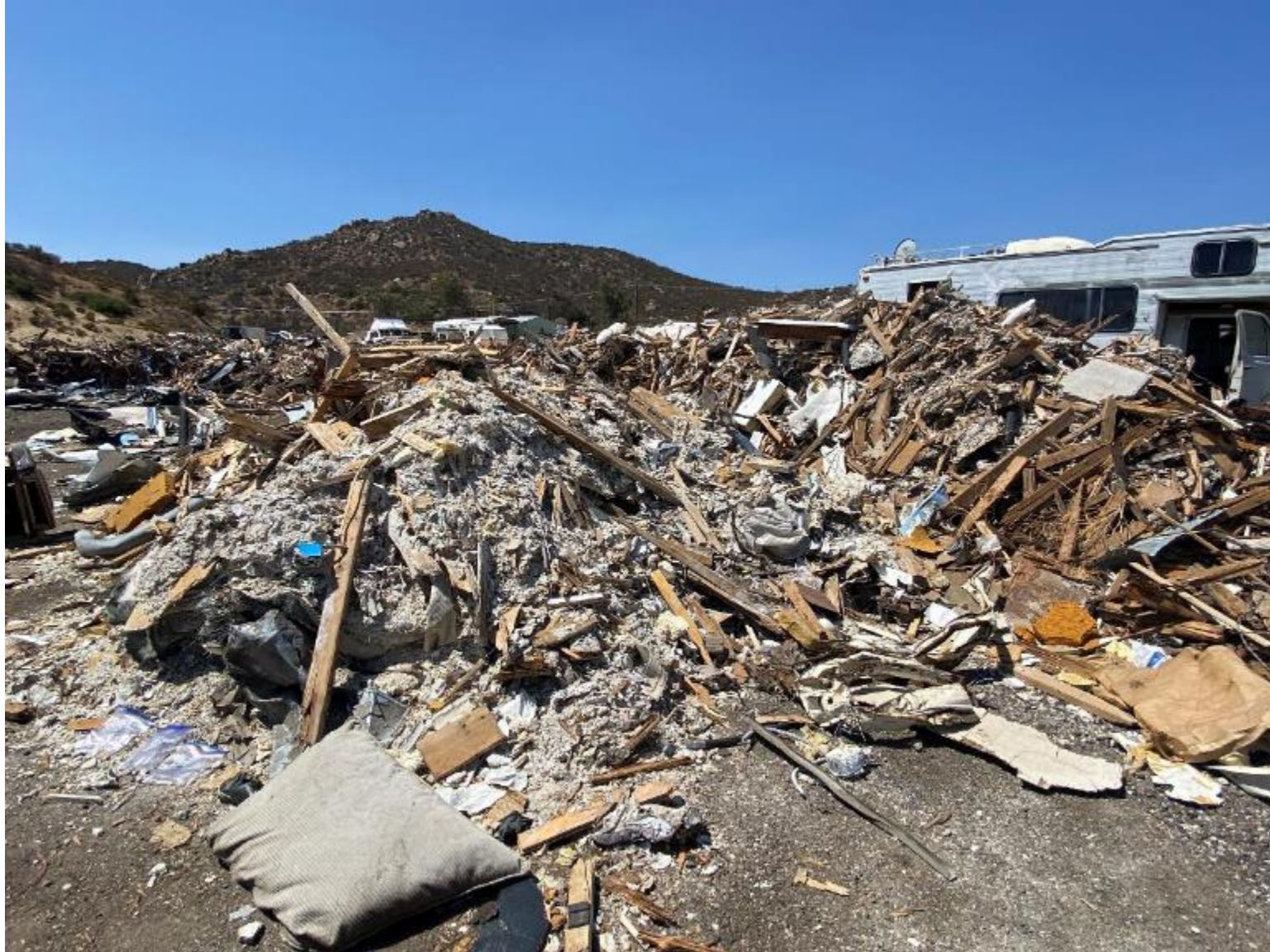
Potential ACM in construction debris
